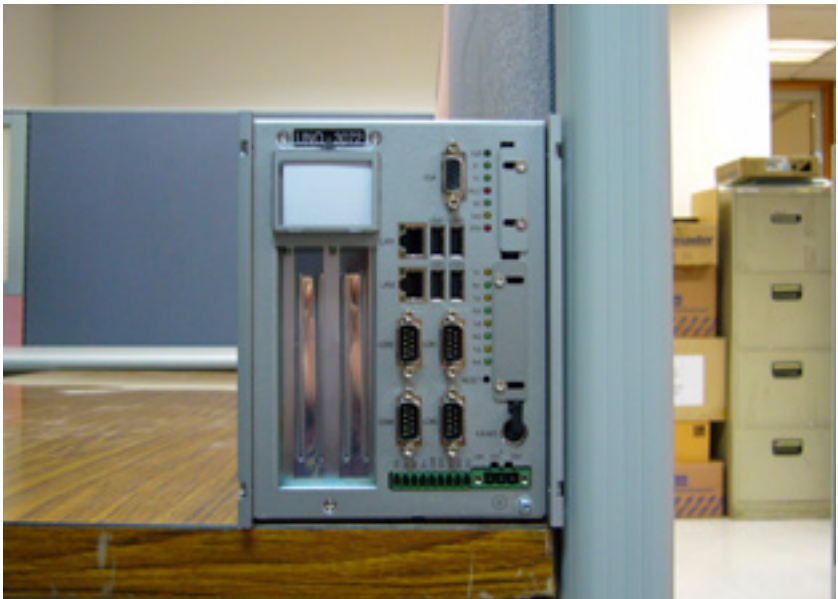
Figure 3.6: UNO-3072 Improper Installation (2)
