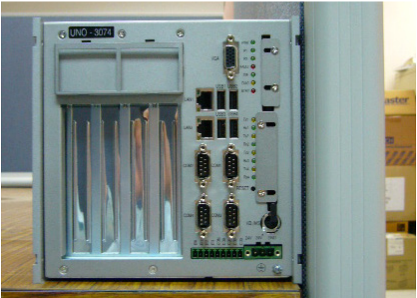
Figure 3.6: UNO-3074 Improper Installation (2)
