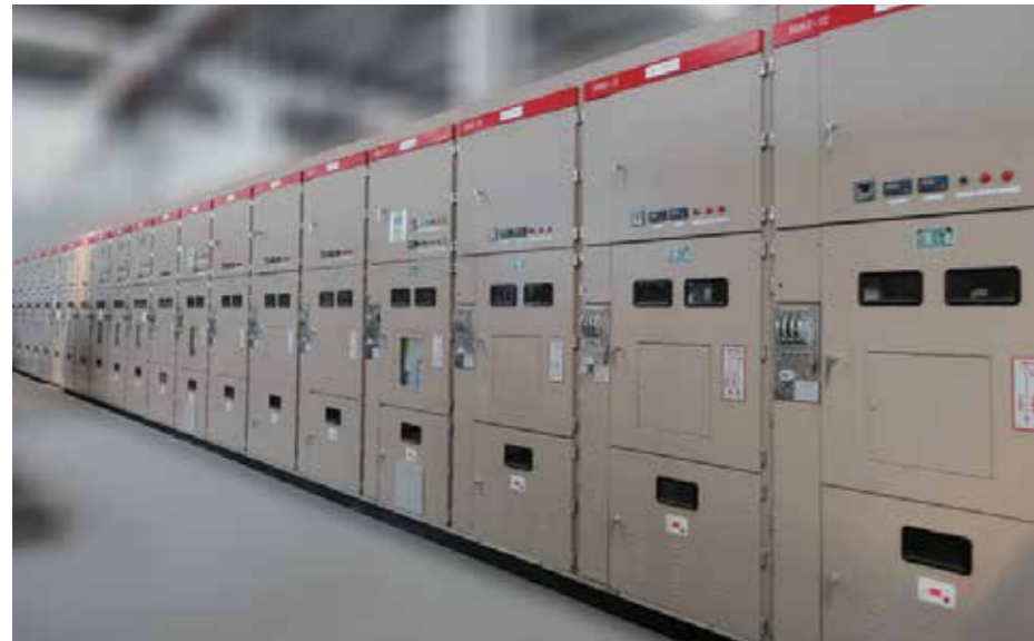
• High Voltage Distribution Cabinet
