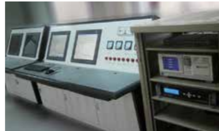
• Central control room
