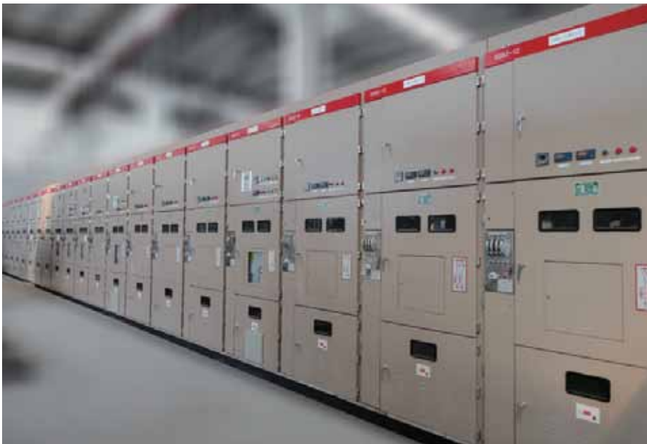
• High Voltage Distribution Cabinet
