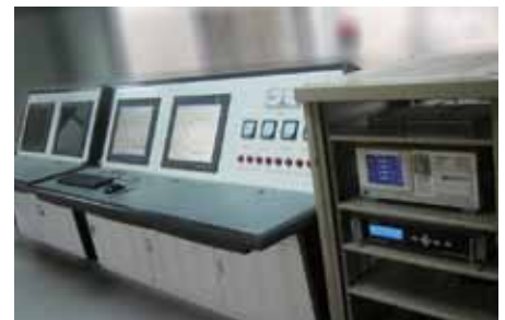
• Central Control Room
